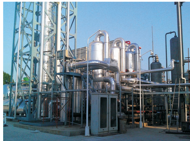
CO 2 Recoverd & Purified Plant (200,000 ton/y)
